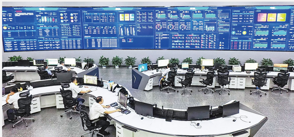
▶ Intelligent Operation Control Center
