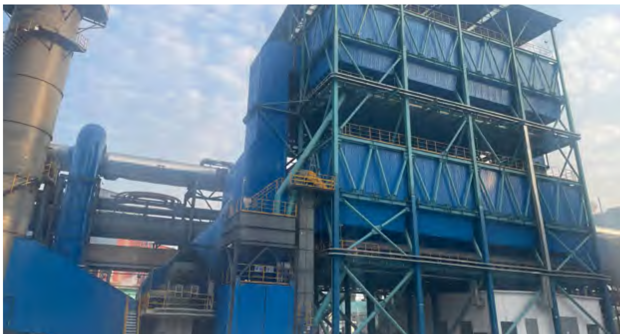
Flue gas desulfurization project of the blast-furnace hot blast stove
