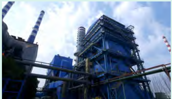
Desulfurization and denitrification of sintering machine flue gas
